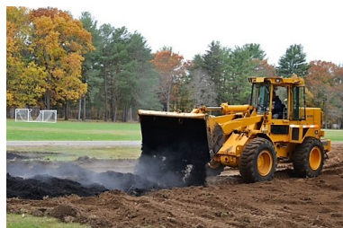
Groundbreaking for Hamilton Wenham GC’s Garden for the Community at Pingree Park
